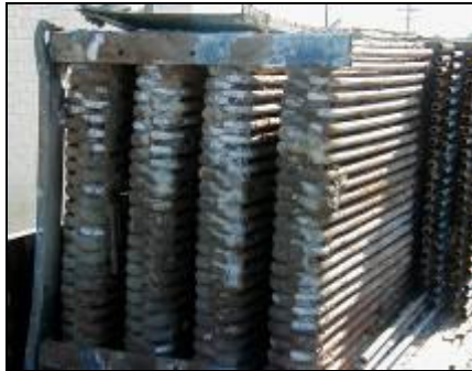
Prohibited: Heat exchanger with deposit / scale
