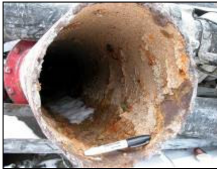
Prohibited: Pipe with radioactive deposit / scale
