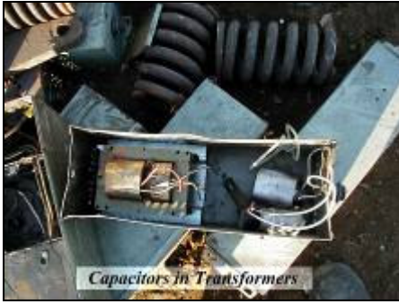
Prohibited: Capacitors in transformer
