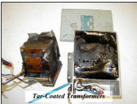
Prohibited: Tar-coated transformer
