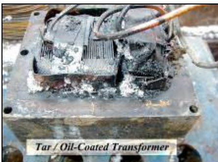
Prohibited: Tar-coated transformer
