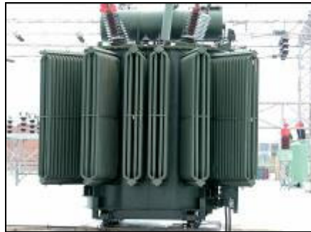
Prohibited: Transformer & components
